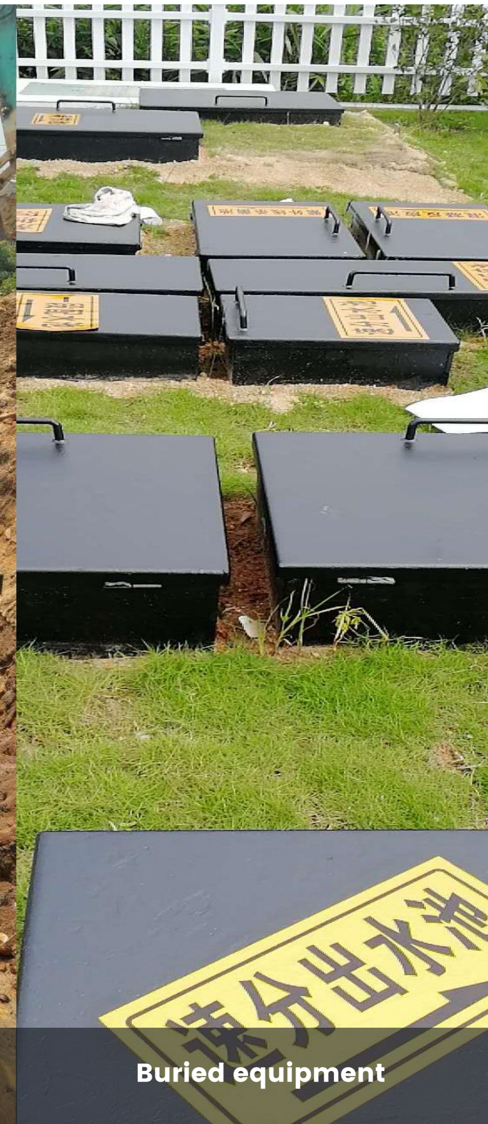
CDT Integrated equipment
